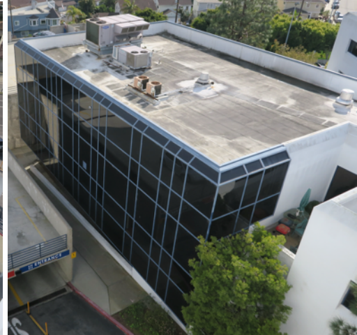
Fig. 11 – 1979 Addition & HVAC Equipment
